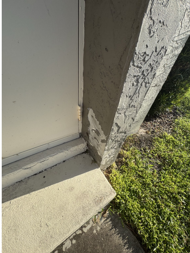
Example of peeling paint to remove during preparation. Directly prime any bare stucco where old paint is removed.
