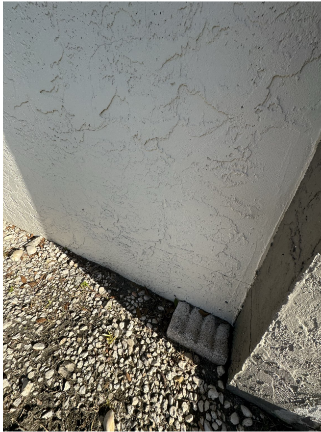
Example of stucco settling cracks to elastomeric fill and seal.
