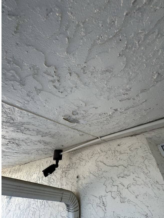
Example of peeling paint to remove during preparation. Directly prime any bare stucco where old paint is removed.
